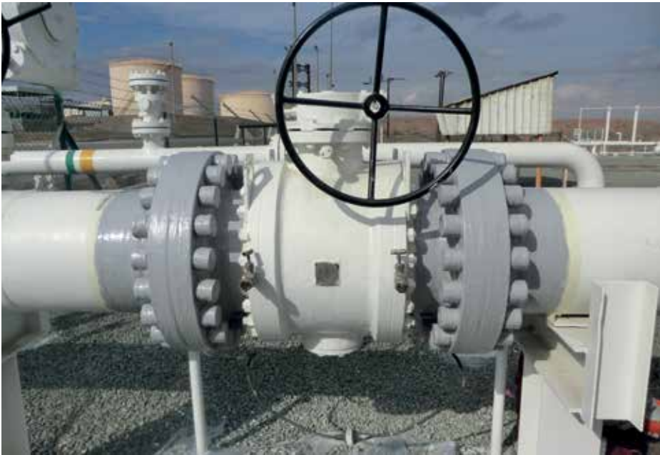
Left: Belzona 3411 successfully installed on over 500 flanges with different shapes and configurations
