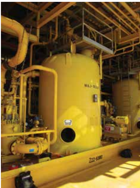
Above: Leaking seawater filter vessel
